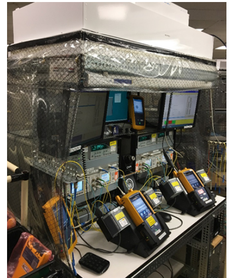
Figure 2 - Fiber calibration station. Note the plastic around the station on the filtration system on top to reduce dust. Some of the commercially available products used are modified by Fluke Networks to meet our accuracy requirements.
